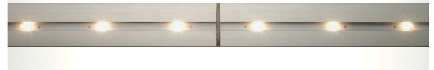
Shard undercabinet wiring
